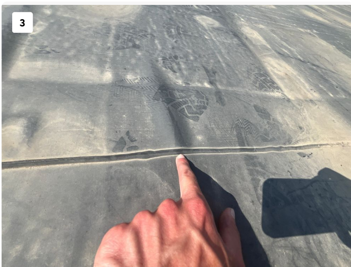
All seams have been addressed with an adhesive. Adhesive is holding up well and saw no gaps or cracks.
