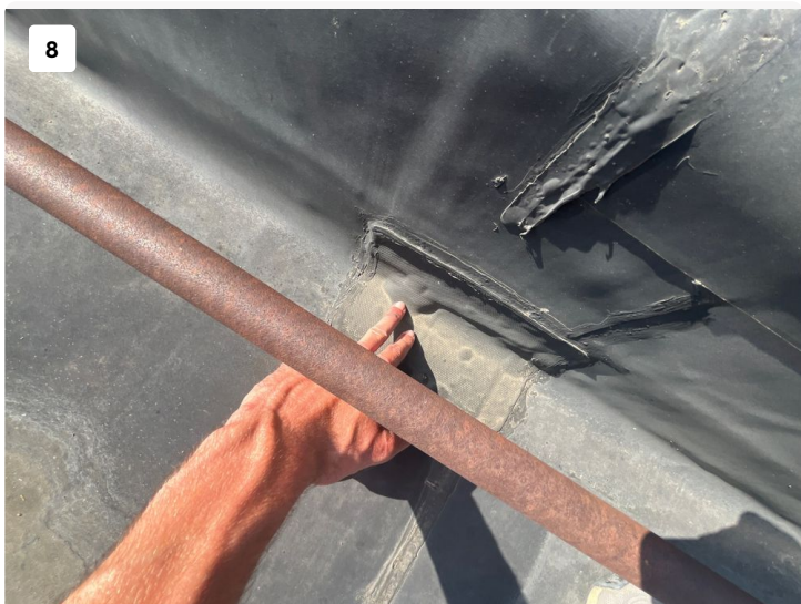
Air bubble underneath EPDM patch.
