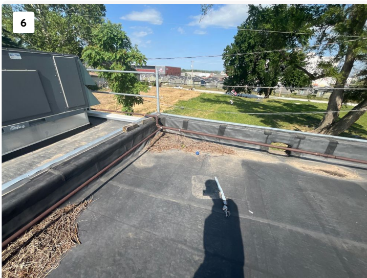
Debris on the roof near the scupper. This should be removed.
