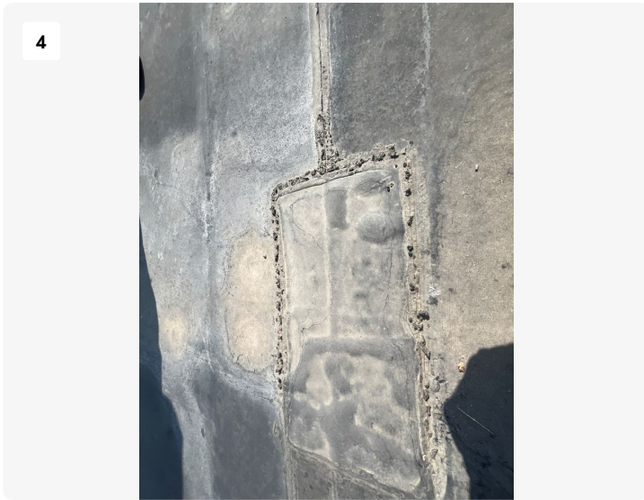
Deteriorated seams around EPDM patch. There are also small bubbles forming underneath EPDM.
