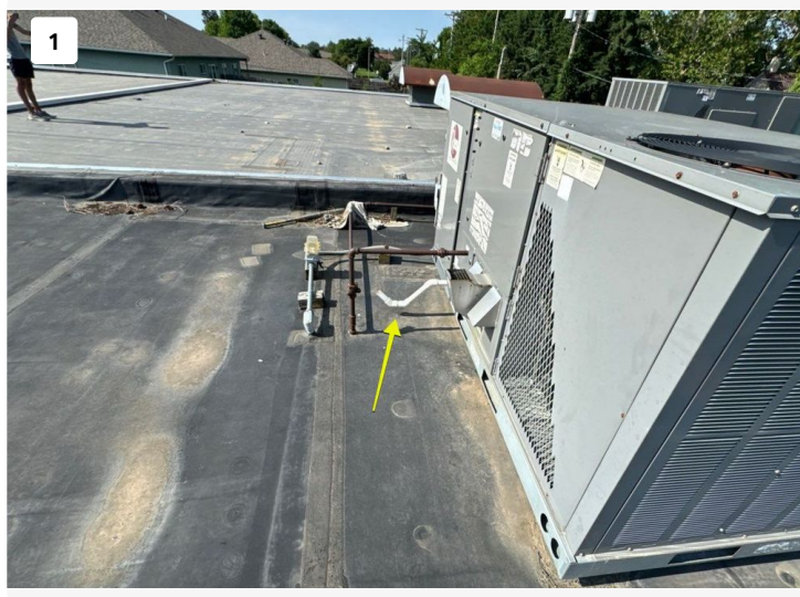
Condensation line not ran to gutter.
