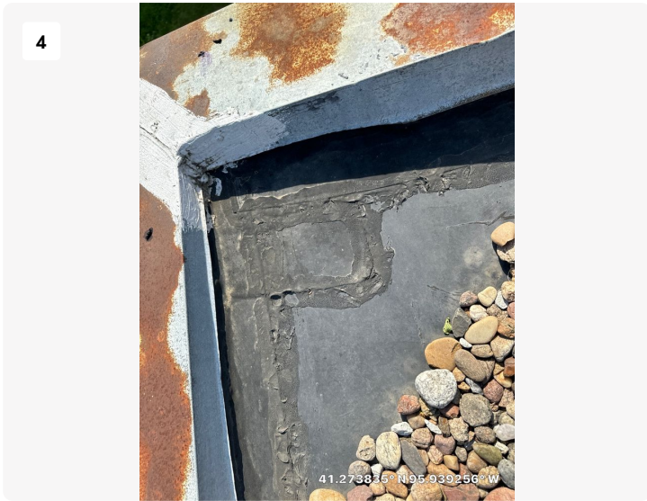
Membrane tenting in the corner. Adhesive is holding up fine but could begin to fail soon.
