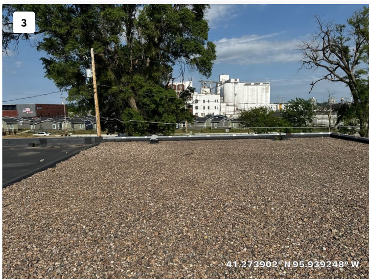
Rooftop vent has minor patch failure.
