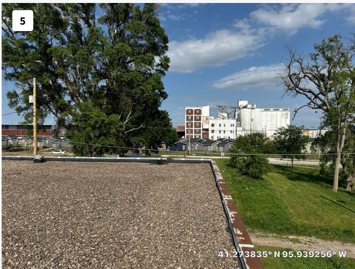
Roof slopes to the East wall well. Water does not pond on this roof.
