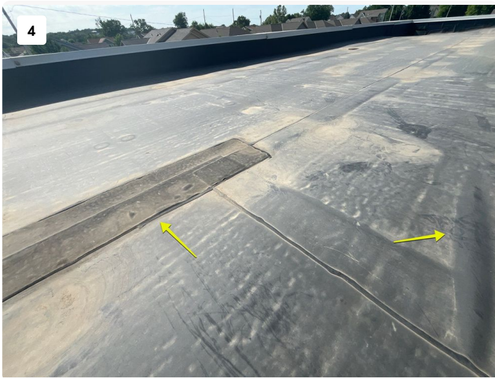
Slight wrinkle in the membrane.
