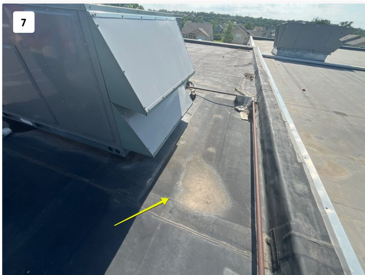
Minor ponding water near an RTU.
