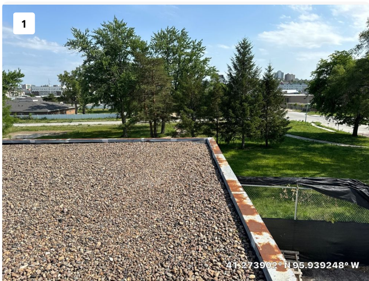
Rusted metal flashing around entire perimeter.
