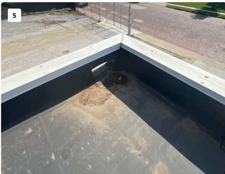
Roof 1 has two scuppers that the roof slopes toward on the northwest and southwest side. Minor ponding water area near scupper.
