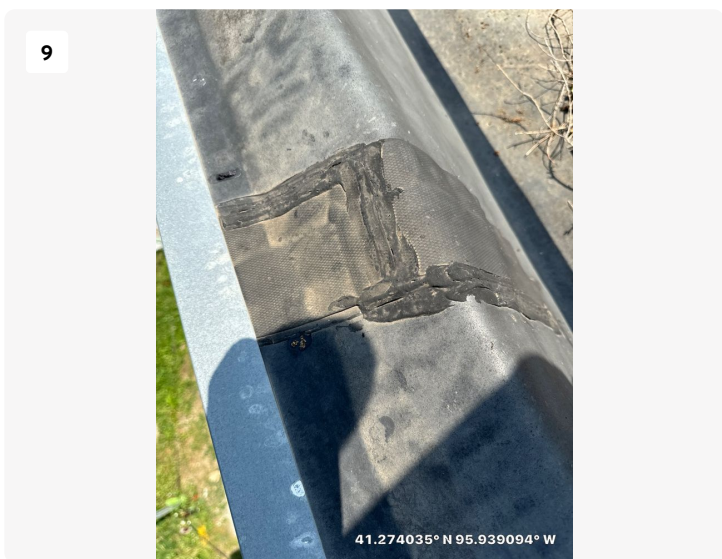
Failing adhesive around EPDM patch.
